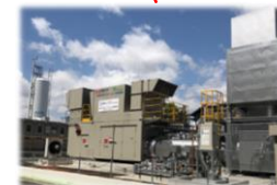
Hydrogen power generation & Heat supply
